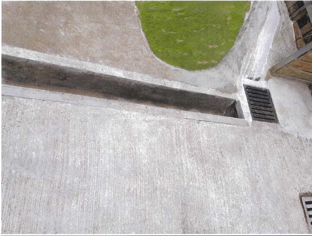
Photo (1) : The terminal catchpit
